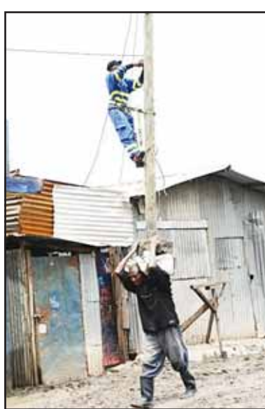
An engineer works on a power line pole in Nairobi, Kenya on May 6. The number of people who have lost their lives in the devastating floods and landslides triggered by heavy rains in Kenya since March has risen to 238, with 75 others still missing, the government said on May 7. (Xinhua)
