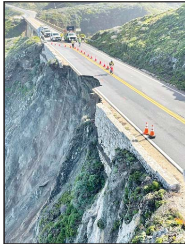
This photo provided by Caltrans shows a damaged section of Highway 1, on March 31, south of Rocky Creek Bridge in Big Sur, Calif. Authorities urged motorists to avoid the scenic highway after a section of the coastal route collapsed during an Easter weekend storm, forcing closures and stranding motorists near Big Sur, authorities said. (AP)
