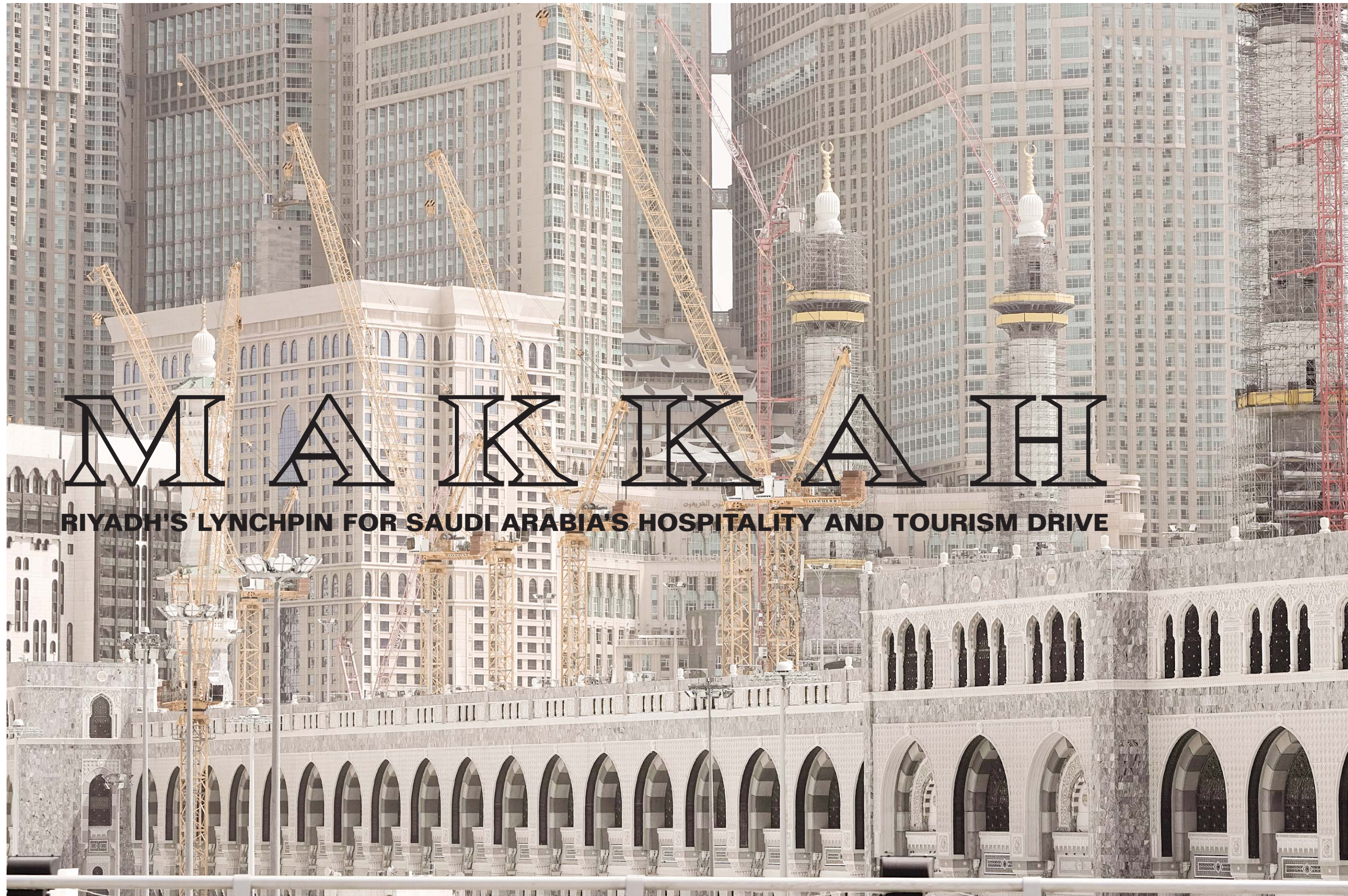
Cranes are seen on the new extension of the Grand Mosque during the Hajj pilgrimage in the Muslim holy city of Makkah, Saudi Arabia, Sunday, June 25, 2023. Saudi Arabia is pumping billions of dollars into the holy city of Makkah to meet its ambitious economic targets, with high-end hotels, apartment blocks, retailers and restaurants planned for areas around the Grand Mosque. (AP)
