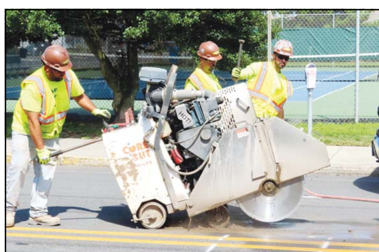
A worker uses an industrial cutting machine to open a section of the street in Ocean City, N.J. on Sept. 12, 2023, at the start of land-based probing along the right-of-way where a power cable for New Jersey's first offshore wind farm is proposed to run. Federal regulators have determined that plans for Orsted's wind farm off Ocean City are not expected to kill or seriously injure marine life. (AP)
