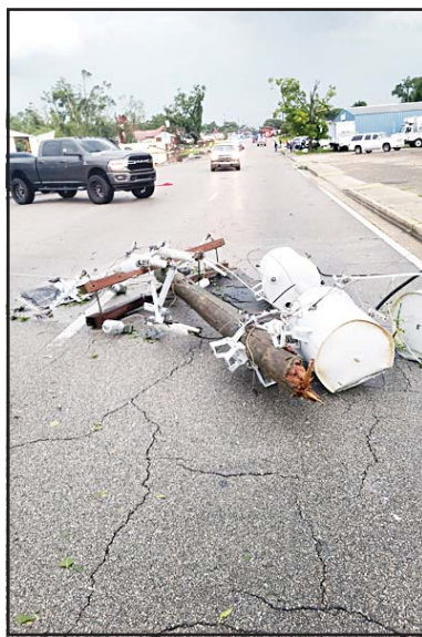
A power transformer sits in the street in Moss Point, Miss., after a tornado struck the area, Monday, June 19. (AP)
