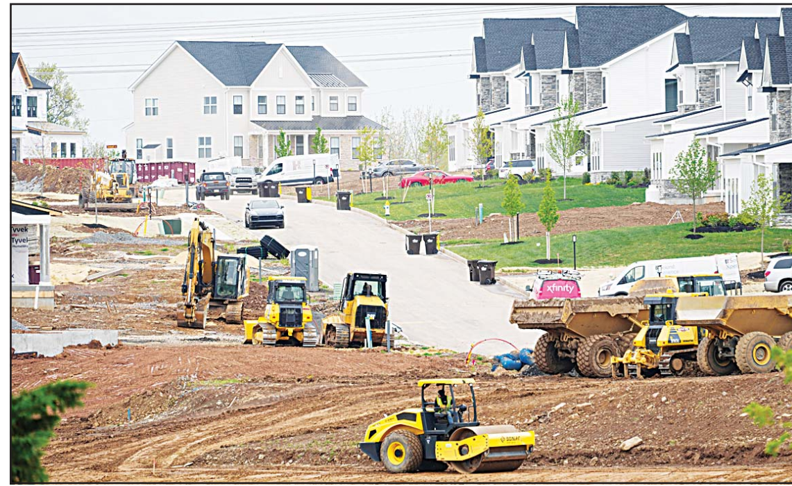
A residential development under construction in Eagleview, Pa., Friday, April 28, 2023. Homebuilders are stepping up construction of single-family homes following a steady decline in mortgage rates and broad expectation among economists that home loan borrowing costs will ease further in 2024. (AP)
