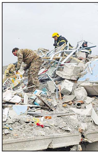
This photo released by Belgorod region governor Vyacheslav Gladkov's telegram channel on, March 18 shows emergency ministry employees working at the destroyed building after shelling from the Ukrainian side, in Nikolskoye village, Belgorod region, Russia. Russia plans to evacuate about 9,000 children from a border region because it is being shelled continuously by Ukraine, an official said on March 19. (AP)
