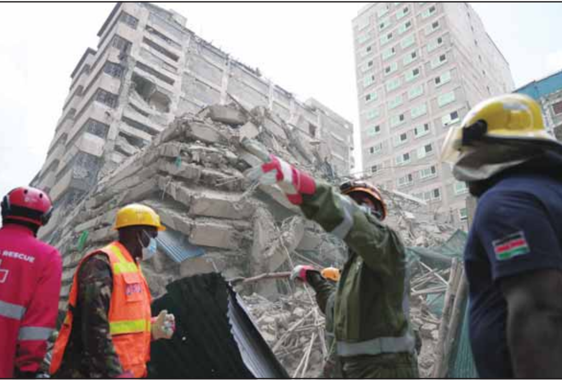
Security forces and civil defense work after a multi-story building collapsed in Nairobi, Kenya on Oct 23. (AP)
