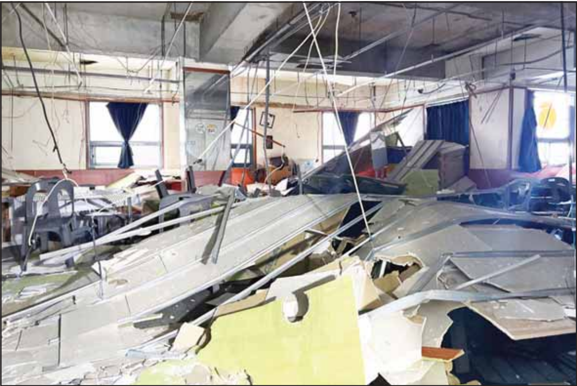
A general view of a scene after parts of a plaster ceiling collapsed at a building in Daegu, South Korea on Oct 10. (AP)
