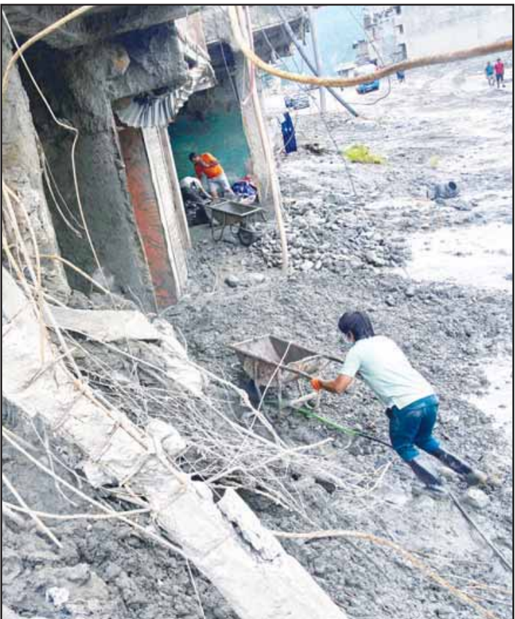
A worker clears mud from a house damaged by flash floods at Nuwakot, Nepal on Sept 23. (AP)
