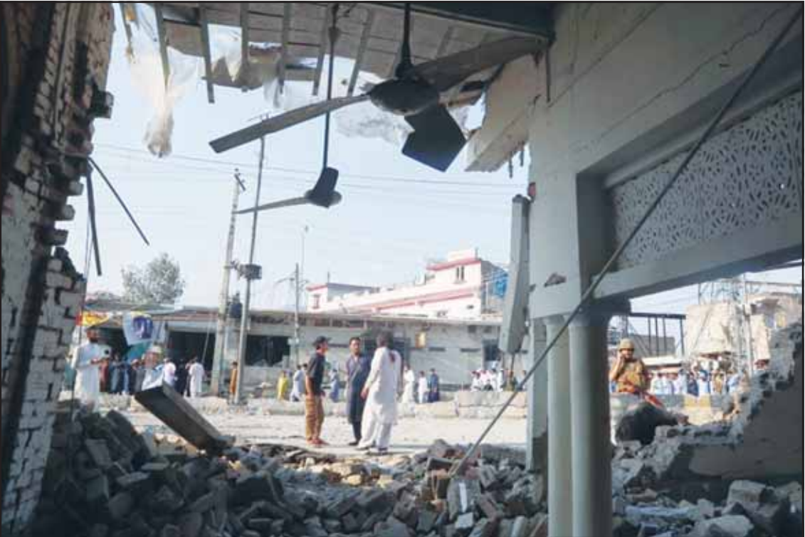
An Army soldier and local residents look at a damaged portion of a mosque after a bomb exploded in Kohat, in northwestern Pakistan on Sept 18. (AP)
