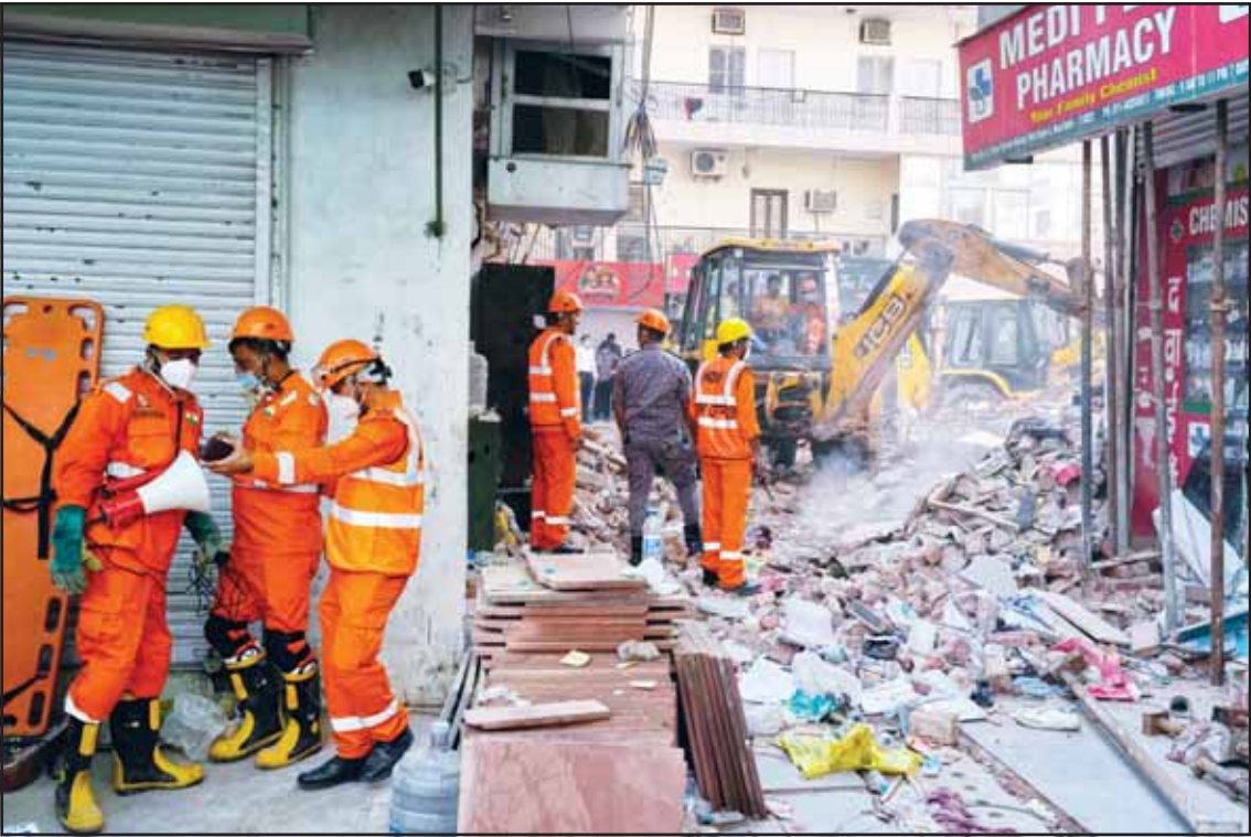
Rescuers clear debris as they search for people possibly trapped at the site of a collapsed building in New Delhi, India on Sept 7. (AP)
