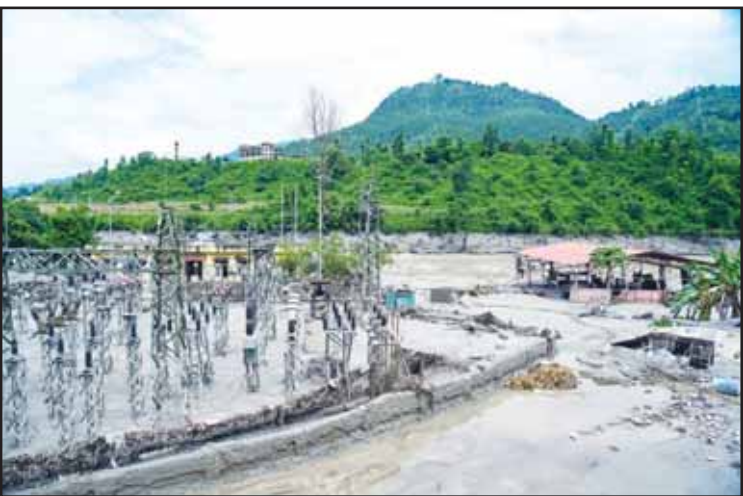
An electrical equipment at a power plant is partially buried in slush brought in by the Trishuli river in flash floods, in Dhading District, Nepal on Aug 30. (AP)
