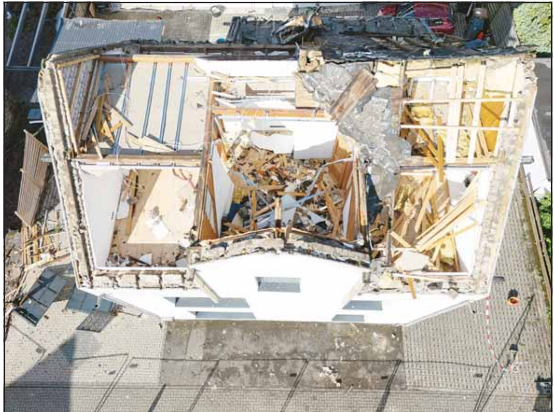
Severe damage is visible on several houses in Solms-Oberndorf, Germany on Aug. 20, 2026, following a violent thunderstorm. (AP)
