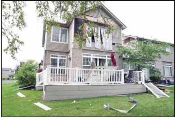
A home is damaged after a storm in Tinley Park, Illinois on Aug 11. (AP)
