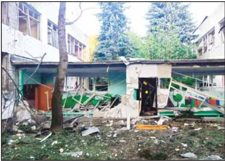
This photo, released by Moscow Region Governor Andrei Vorobyev’s official telegram channel, shows a building damaged during a Ukrainian drone attack in Elektrostal, Moscow region of Russia, on July 18. (AP)
