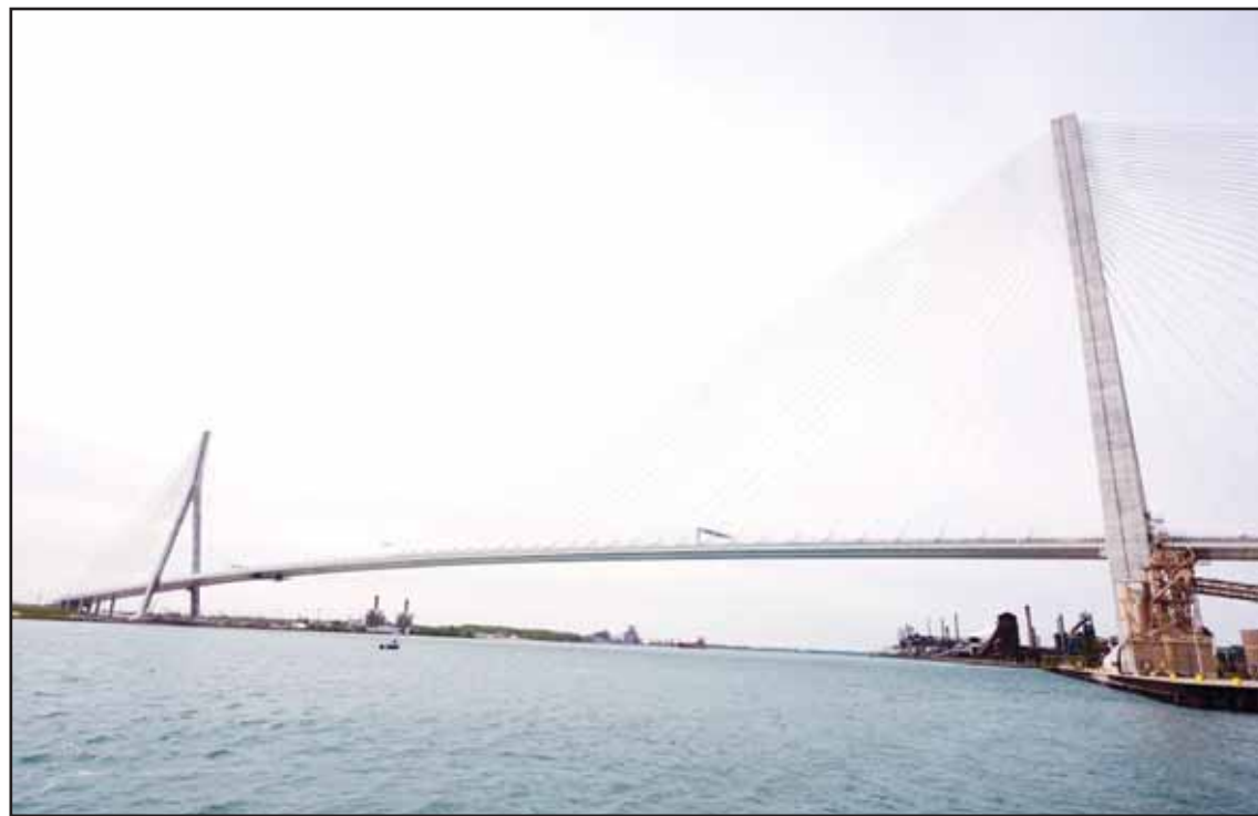
The Gordie Howe Bridge is shown under construction between Windsor, Ontario and Detroit, May 22, 2026. (AP)
