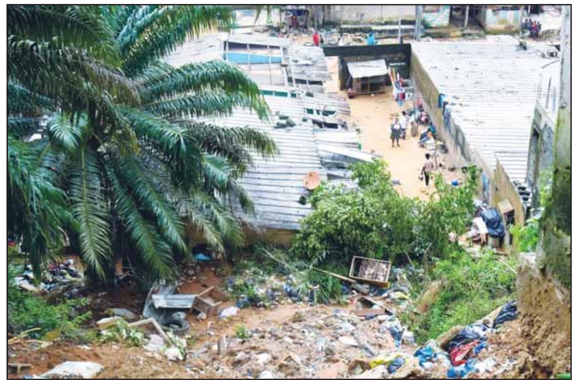
A view of the houses damaged by landslides in an informal settlement of Attecoubé, in Abidjan, Ivory Coast on June 30. (AP)
