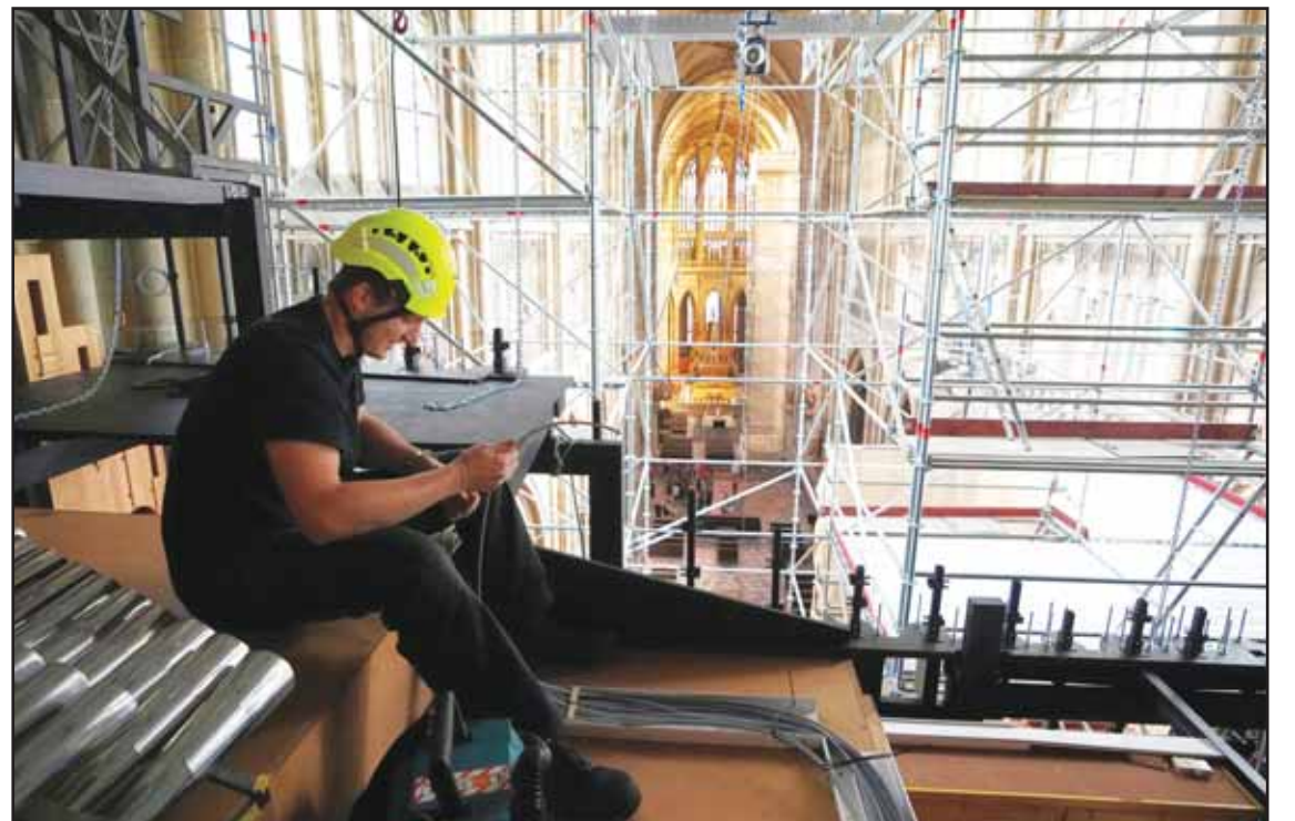
In this file photo, a worker adjusts cables during the installation of a new organ at Prague's St. Vitus Cathedral that is coming to its final stages in Prague, Czech Republic. (AP)
