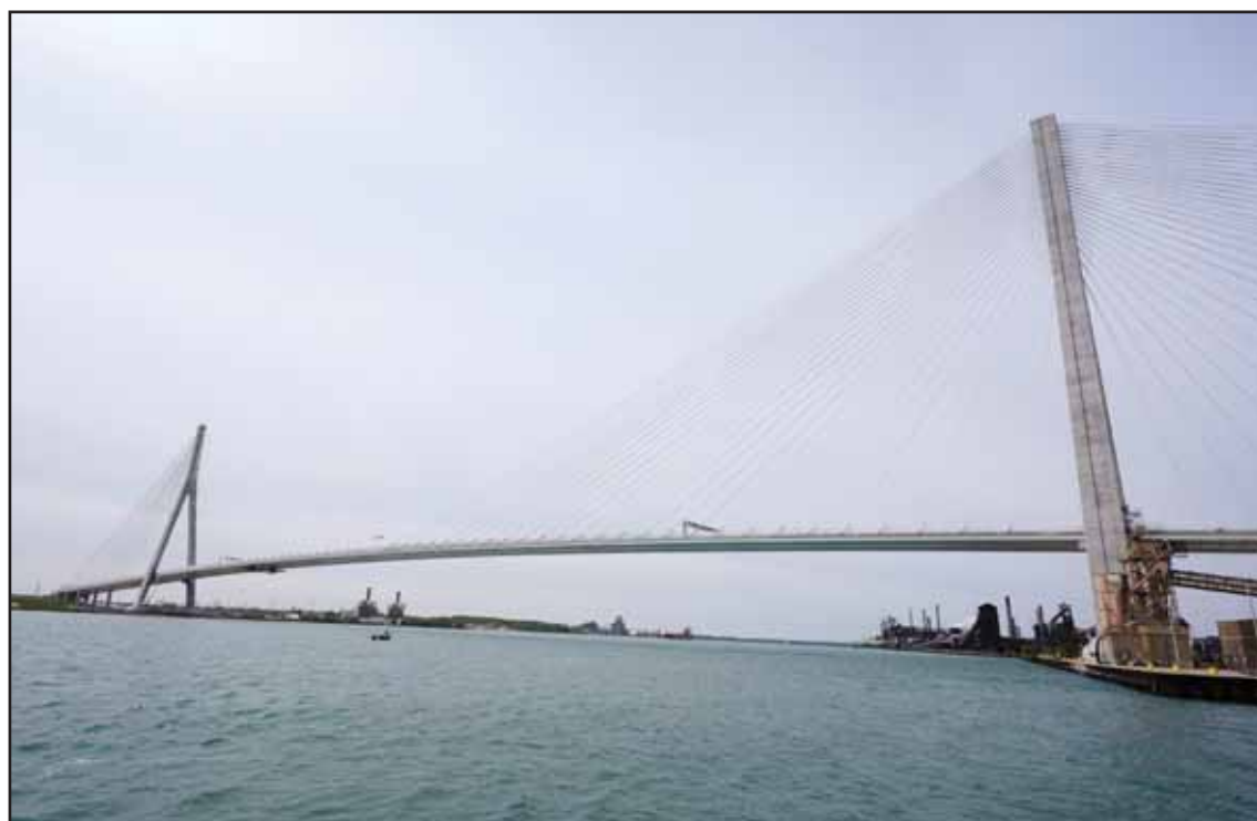
The Gordie Howe Bridge is shown under construction between Windsor, Ontario and Detroit on May 22. (AP)
