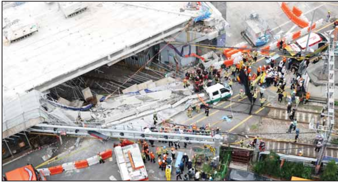
South Korean firefighters and rescue team try to search at the overpass collapsed while it was being dismantled in Seoul, South Korea on May 26. (AP)
