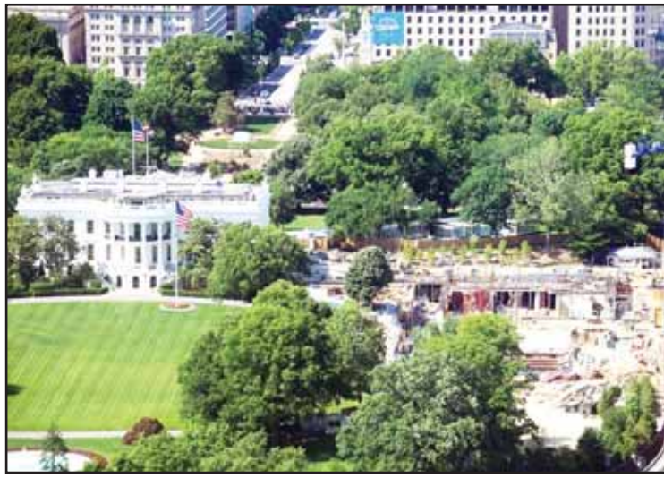
Work continues on the construction of the ballroom at the White House on May 16, in Washington, where the East Wing once stood. (AP)
