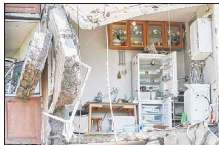
Apartment interiors are seen in a damaged residential house following Russian missile attack in Kyiv, Ukraine on May 14. (AP)
