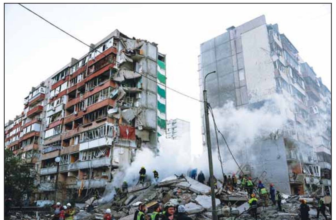
Rescue workers clear the rubble of a house heavily damaged after a Russian strike on a residential neighborhood in Kyiv, Ukraine, on May 14. (AP)
