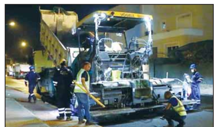
Ministry of Public Works photo Major road maintenance work continues in Mubarak Al-Kabeer Governorate as part of the development plan.
