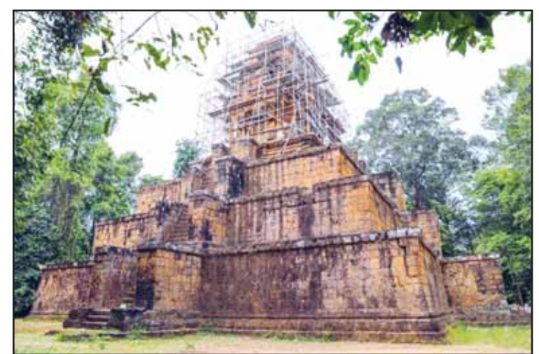
This photo taken on May 8, 2026 shows the Baksei Chamkrong temple in Siem Reap province, Cambodia. Archaeologists have completed the emergency restoration of the early 10th-century Baksei Chamkrong temple in Cambodia's famed Angkor Archaeological Park after parts of the structure were at risk of collapse, the APSARA National Authority (ANA) said in a news release on Saturday. (Xinhua)
