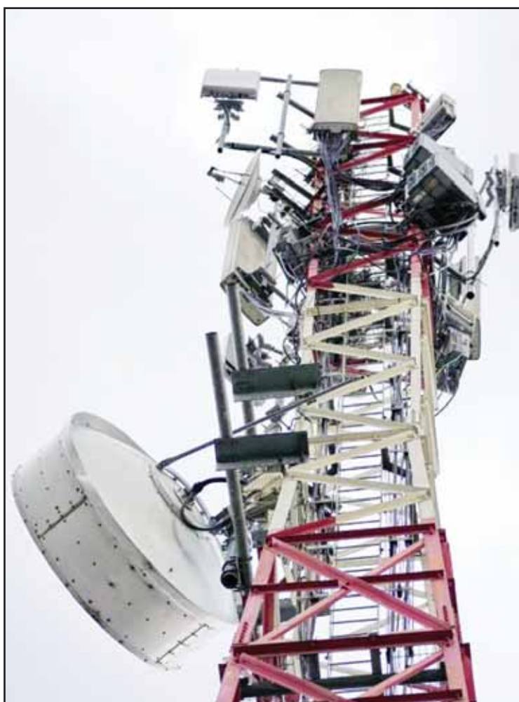
A telecommunications tower stands in Kajjado, Kenya on April 25. (AP)
