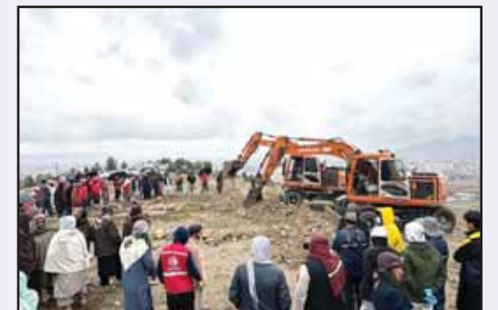
Excavators dig graves for victims of a Monday air-strike on a drug rehabilitation hospital in Kabul, Afghanistan on March 18. (AP)
