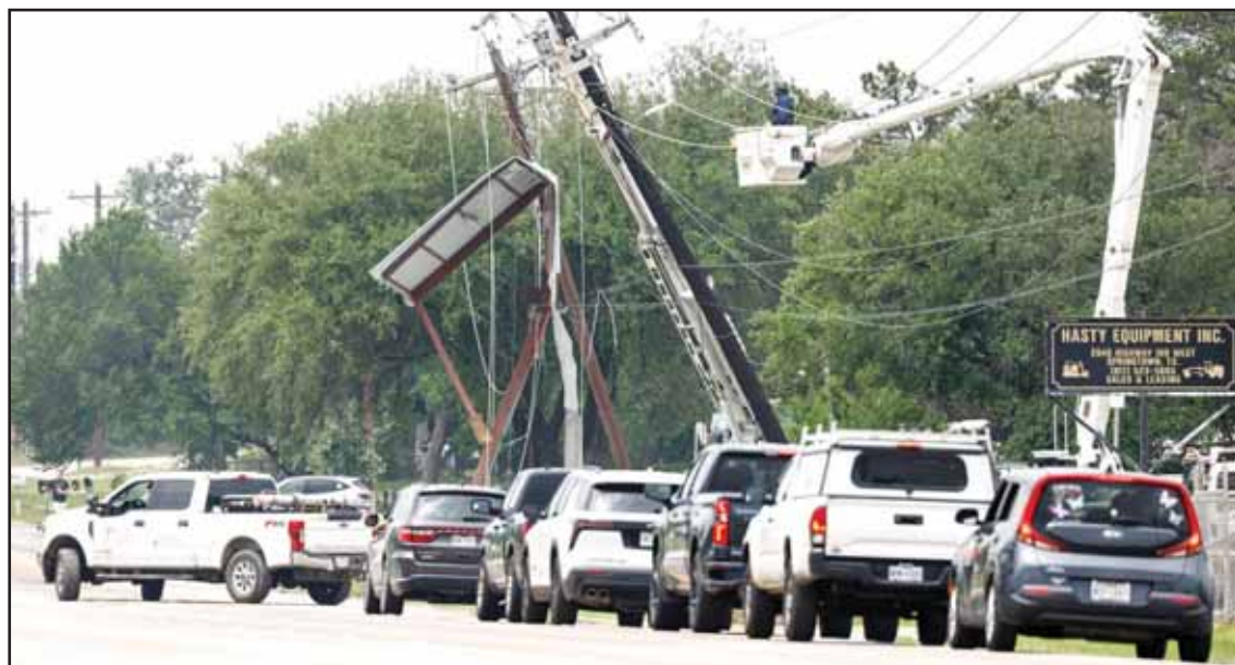
Traffic backs up along State Highway 199 as crews work to repair a heavily damaged power pole and lines along State Highway 199 on April 26, in Springtown, Texas. (AP)
