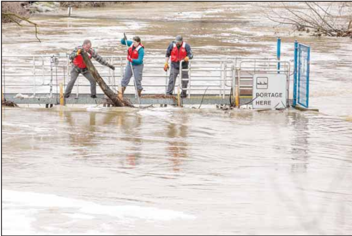
A team of assorted municipality workers clear debris from the Boardman River Weir that was blocking the flow of the flooded Boardman/Ottaway River on April 15 in downtown Traverse City, Mich. (AP)
