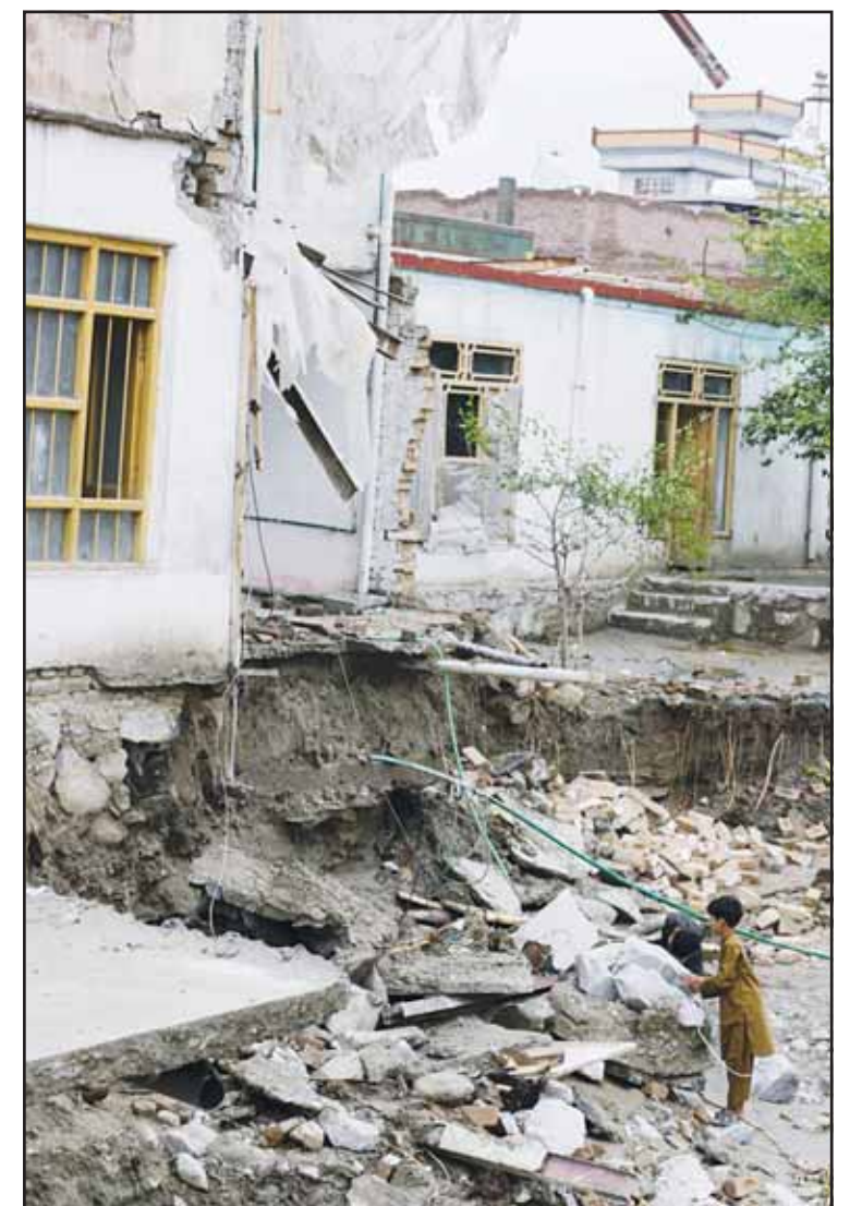
Residents inspect a building that partially collapsed due to heavy flooding in Jalalabad, Afghanistan on April 4. (AP)
