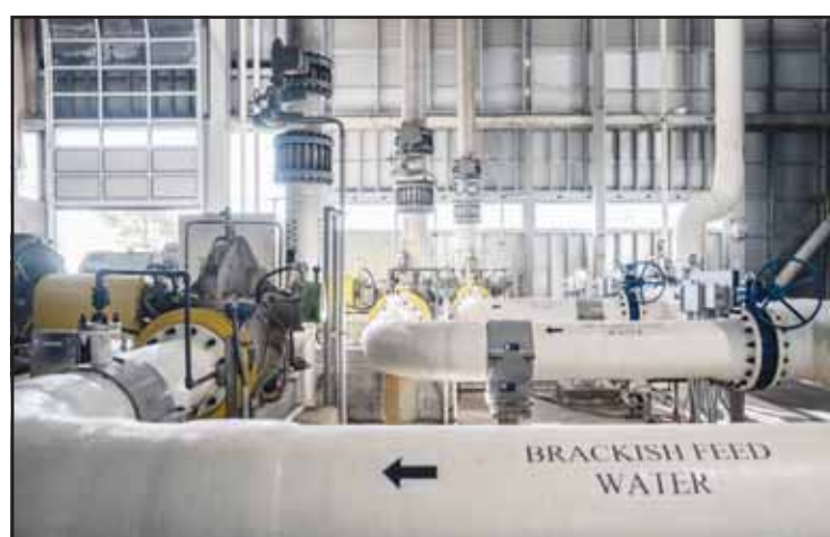
Pipes carrying brackish feed water run through the Carlsbad desalination plant in Carlsbad, Calif., Dec. 2, 2025. (AP)
