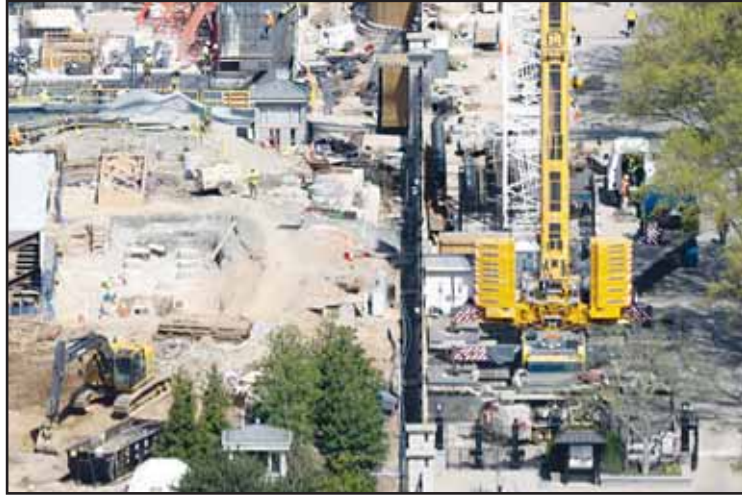
Work continues on the construction of the ballroom at the White House in Washington on April 1. (AP)
