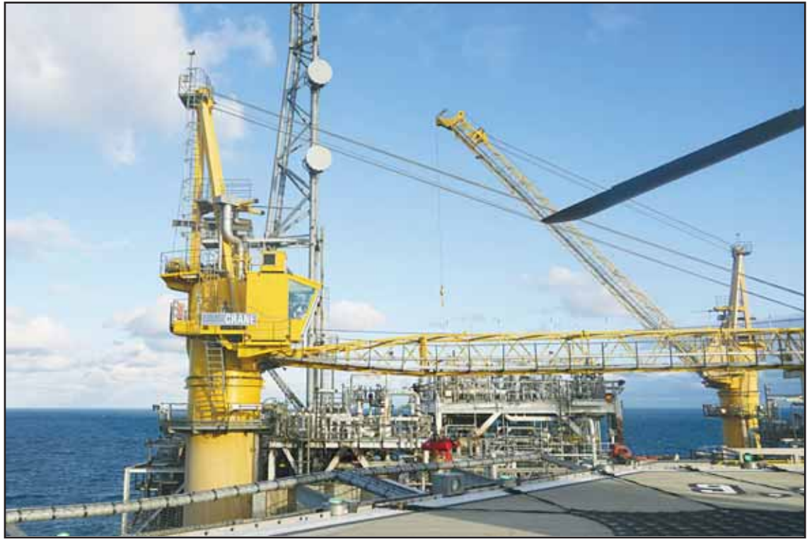
Technical equipment of the INEOS Energy's Siri platform is seen from the helicopter pad at the platform in the North Sea, Denmark, Tuesday, Nov. 25. (AP)
