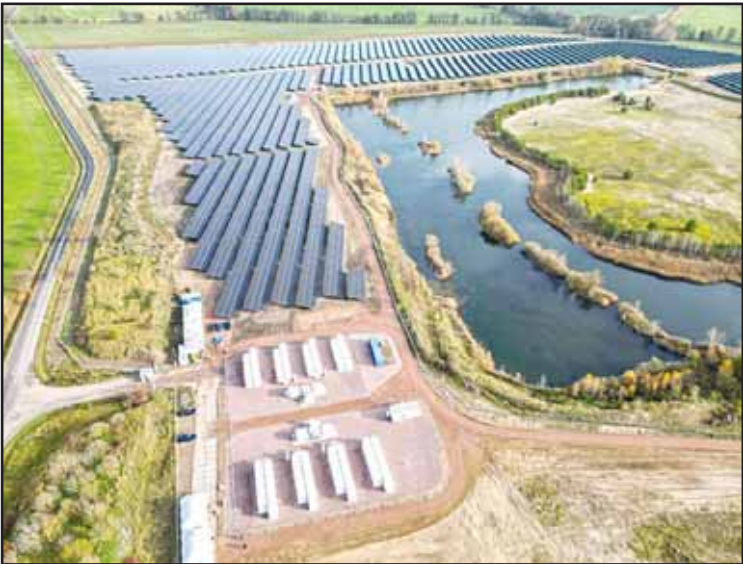
88 battery storage units are located in the new photovoltaic battery storage hybrid power plant on the site of a former gravel pit in Zerbst, Germany, Wednesday, Nov. 12, 2025. (AP)
