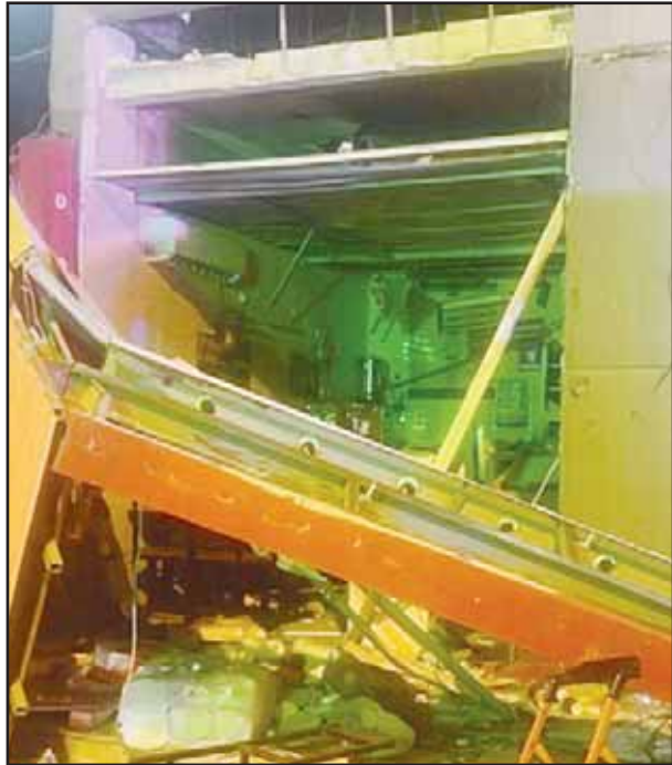
Damage caused by the explosion.
