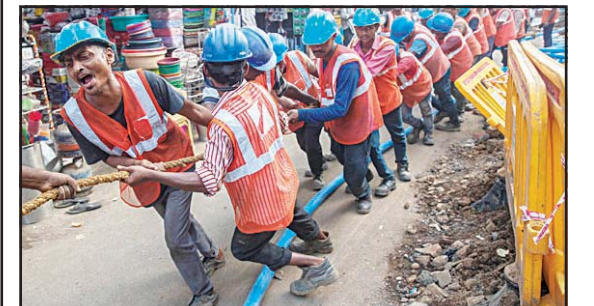
Workers prepare work to lay an underground electricity cable in Mumbai, India Wednesday, Nov. 24, 2021. (AP)
