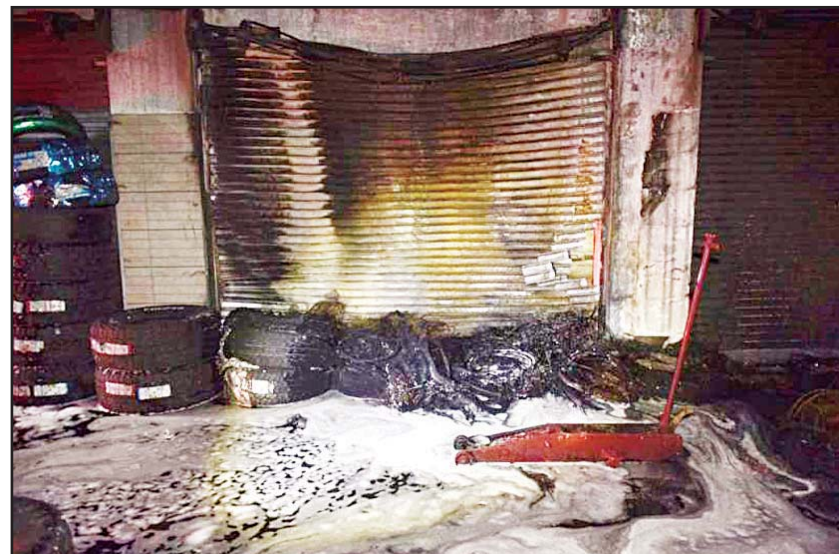
Damage caused by the fire.
