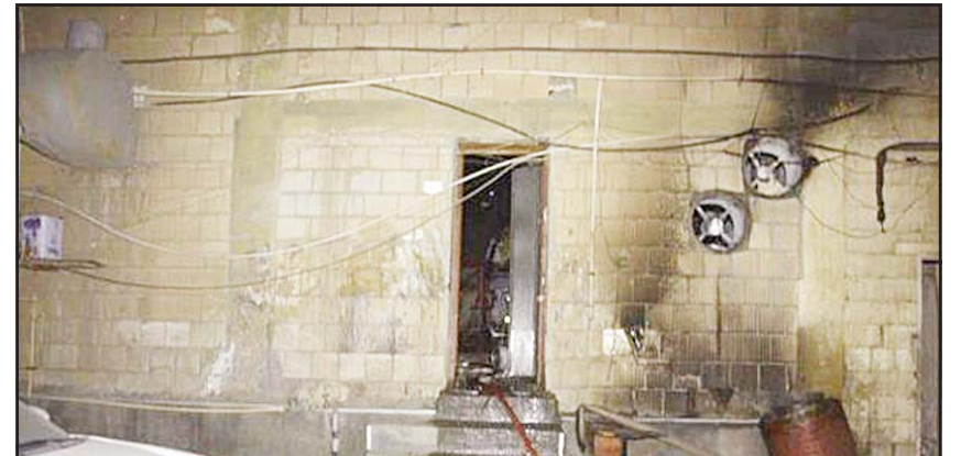
Damage caused by the fire.
