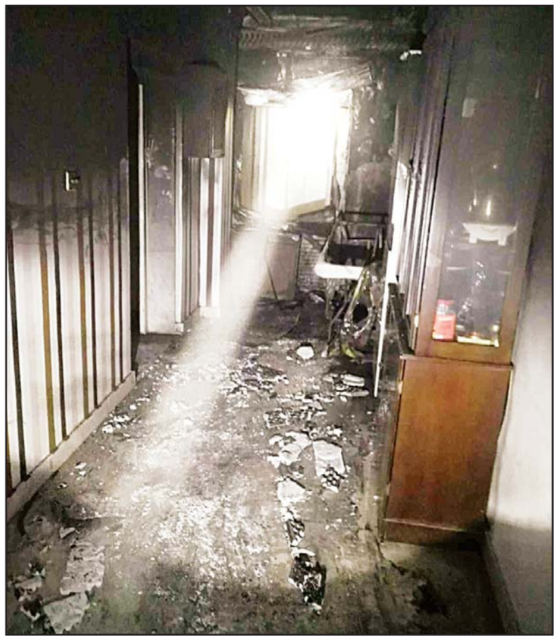
Damage caused by the fire.
