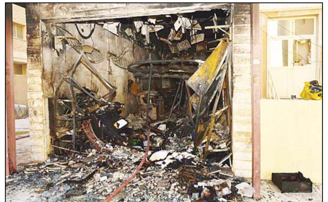
Damage caused by the fire.
