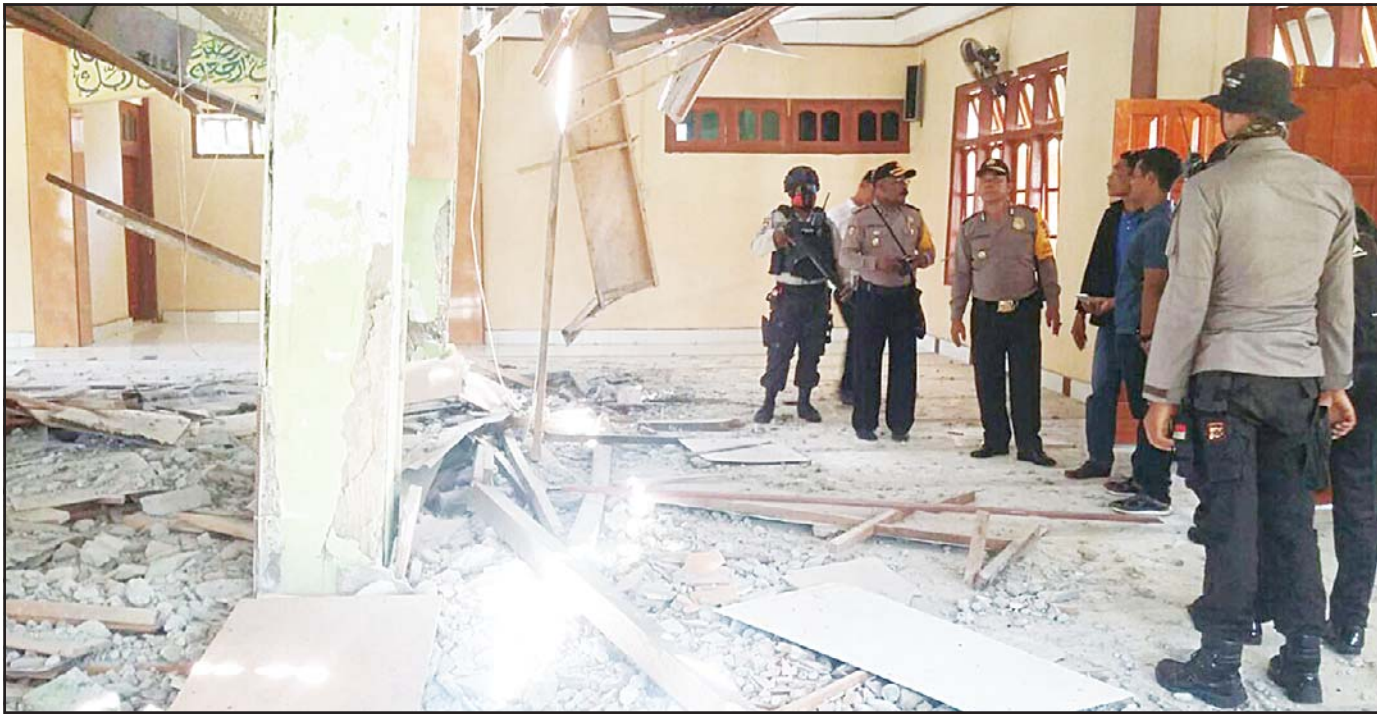
Local officials inspect the damage to a mosque following Monday's powerful earthquake in Papua New Guinea, in Boven Digoel, Papua province, Indonesia. Severe damage to phone networks and roads from the earthquake in Papua New Guinea was hindering efforts to assess the extent of the destruction Tuesday, although officials in the remote central region fear dozens of people may have been injured or killed. (AP)
