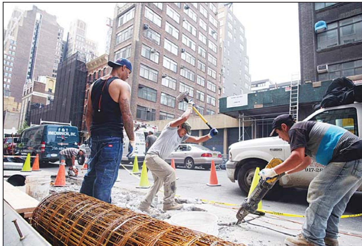
This file photo shows workers as they break a concrete footpath besides a busy street in New York. US construction spending hit a seven-year high in September after a modest rise in the previous month, the Commerce Department reported Nov 2. Despite some signs of slowdown elsewhere in the economy in the month, September
